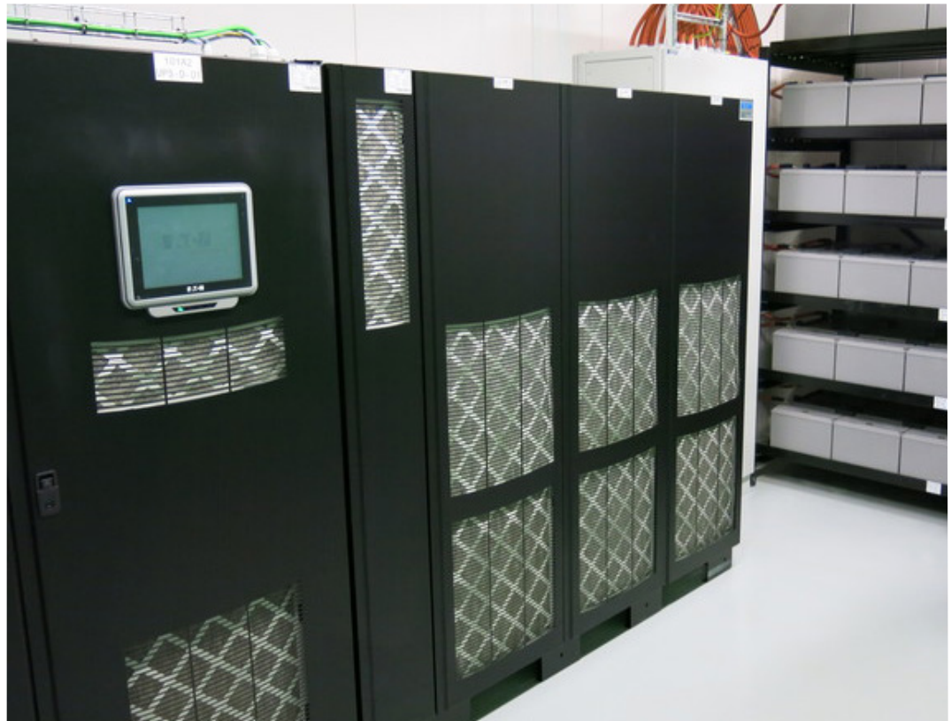
Power Xpert 9395P and batteries
